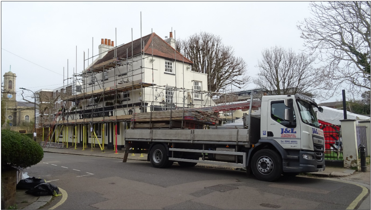
Scaffolding in progress, preparatory for exterior works. Note St Peter's Church to left
